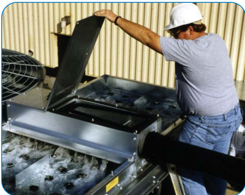
Gravity Distribution Basin
